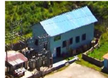
CH Baños I = 0.9 MW
