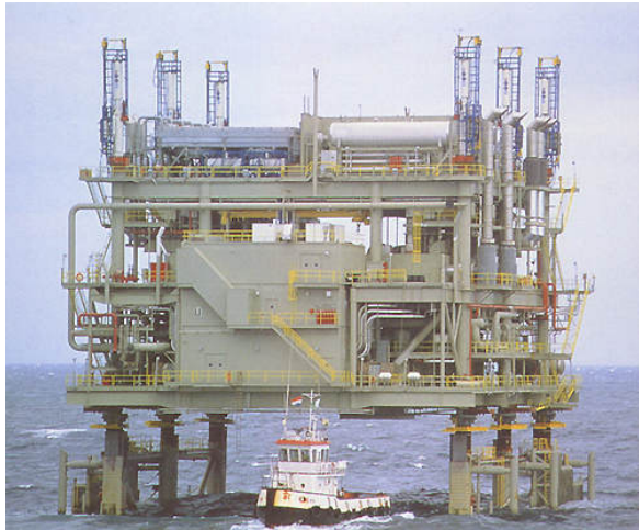
Central Production Platforms
