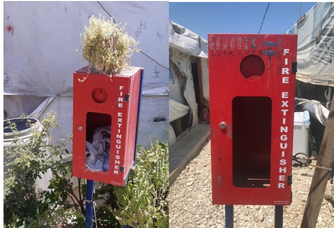
Figures 3 and 4: Empty fire extinguisher boxes, Lebanon 8
