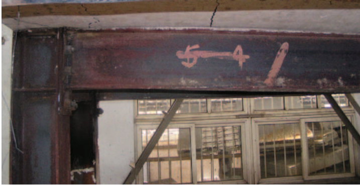
Figure 19. Photograph of the frame at the end of Test 4 showing local buckling of the steel beam. (The color version of this figure is available online.)
