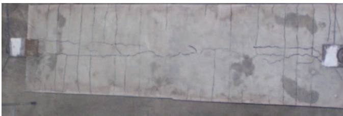
Figure 13. Photograph of the reinforced concrete floor slab at the conclusion of the furnace test. (The color version of this figure is available online.)
