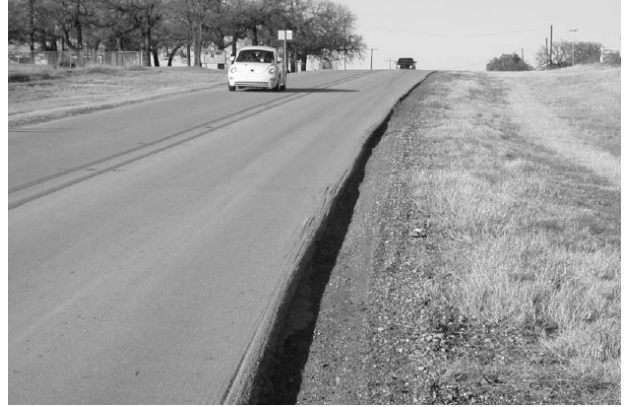
Edge drop-off on narrow roadway (from TxDOT Project 0-4396).
