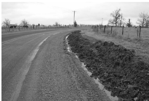
Replenishing repair in progress at inside of horizontal curve (from TxDOT Project 0-4386).
