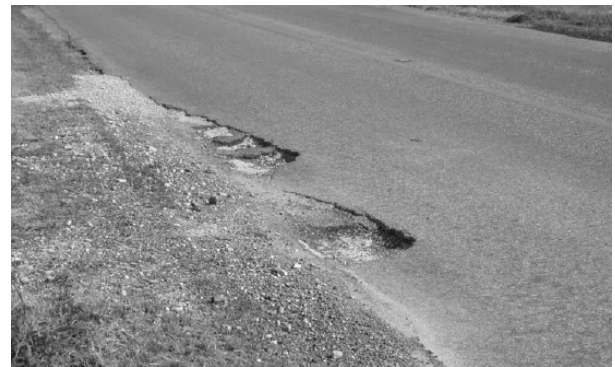
Pavement edge failure (from TxDOT Project 0-4396).
