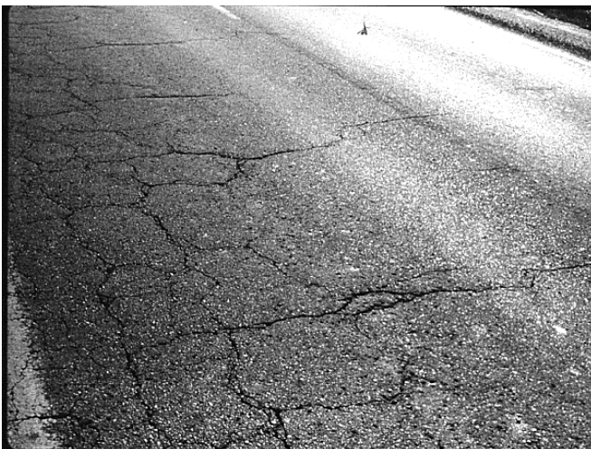
High severity block cracking shown here often is often accompanied by random cracks indicating that the road surface is in an advanced state of deterioration.
