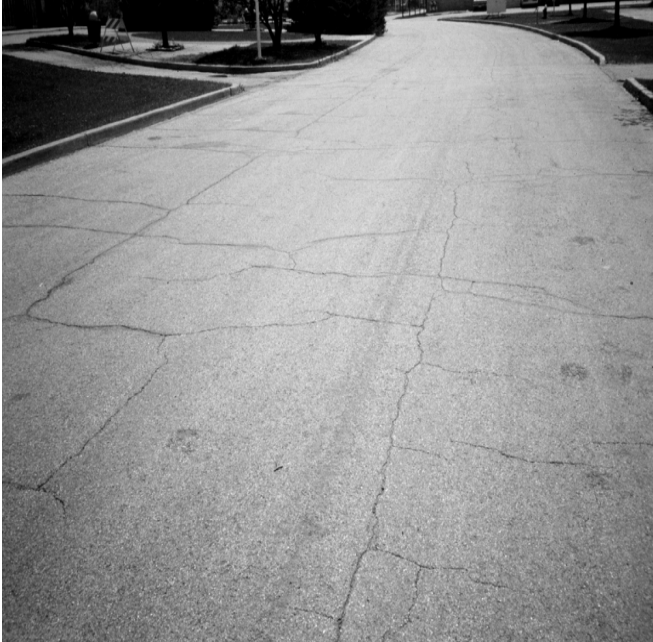
This is an example of moderate block cracking. The cracks are larger than a quarter of an inch and are dividing the pavement into roughly rectangular sections.
