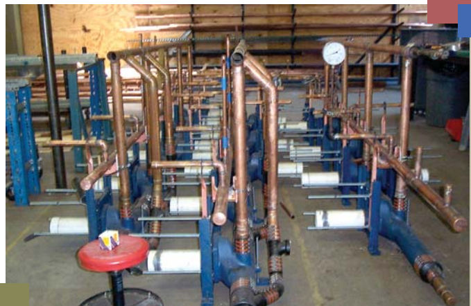
Using drafting and CAD design, piping assemblies are efficiently prefabricated before they are installed at their final location.
