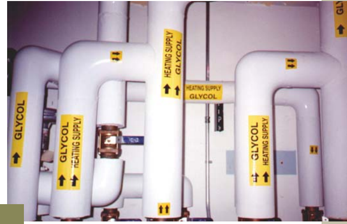
Insulated circulation piping for a heating loop are labeled for easy identification.
