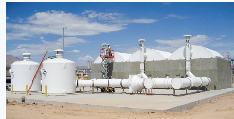
Andronaco Industries recently added a field services offering and expanded its fiberglass vessel/tank and piping capabilities and capacities through acquisition of Diamond Fiberglass Systems and Services in Victoria, Texas.
