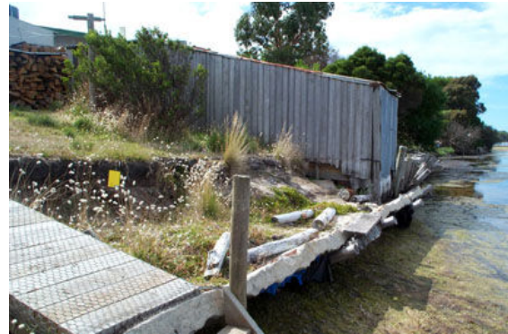
Figure 4: An eroding shoreline at Anson’s Bay (Tas.) in 2002. The wall built to protect the adjacent shacks from erosion has subsequently collapsed and been removed. Photo: C. Sharples
