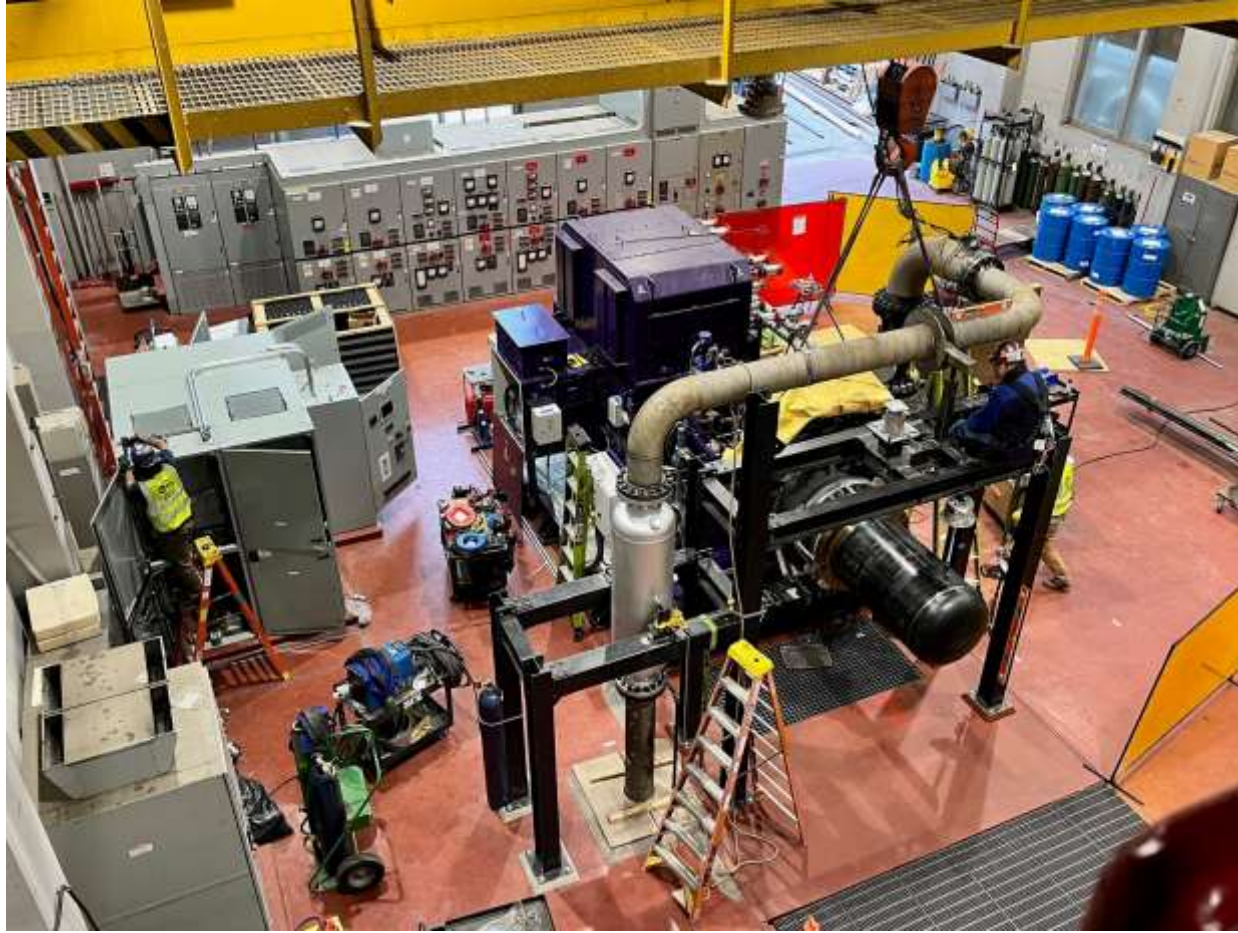
New Switchgear, piping and supports 8/7/2023
