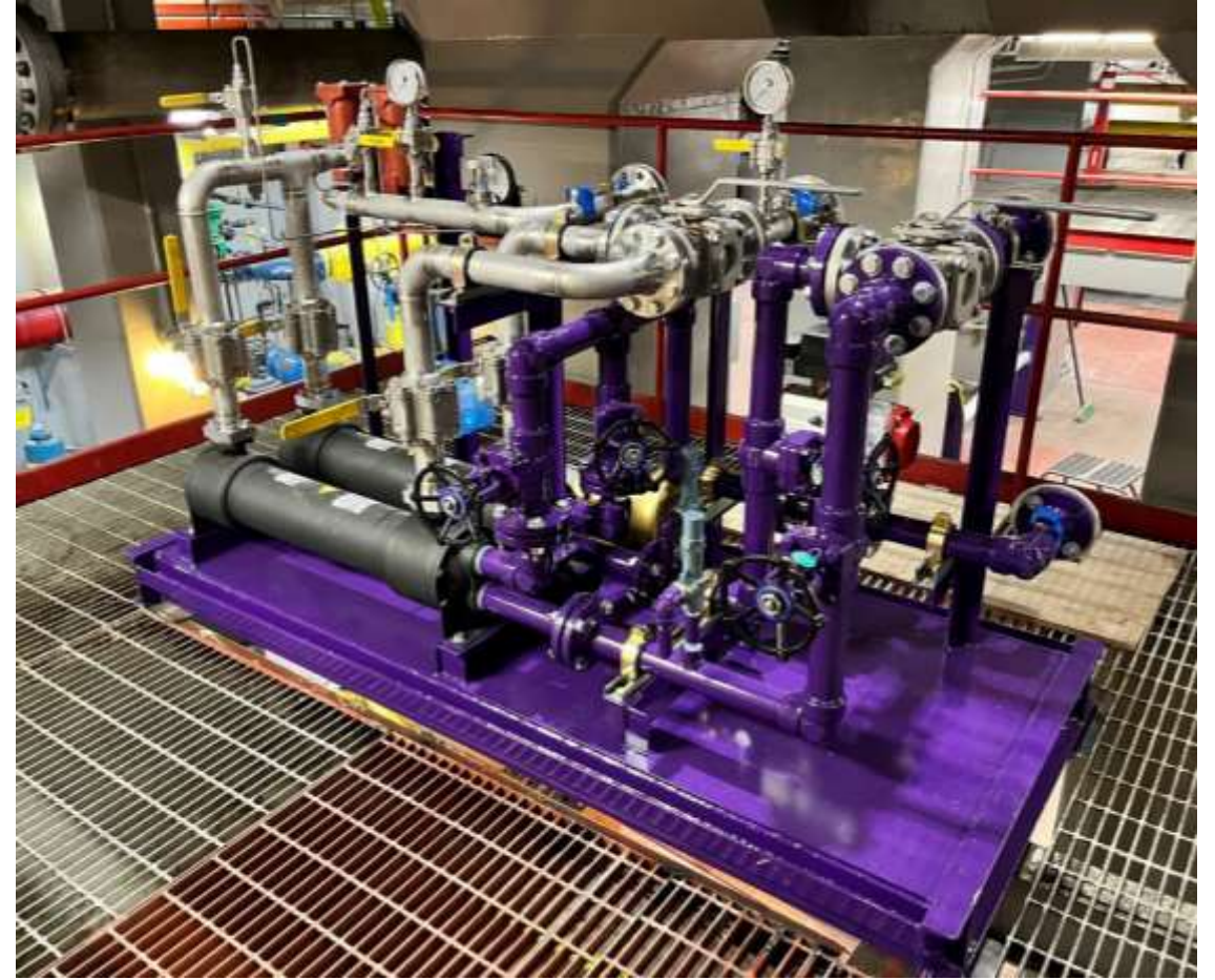
Lube Oil Skid installed 7/3/2023
