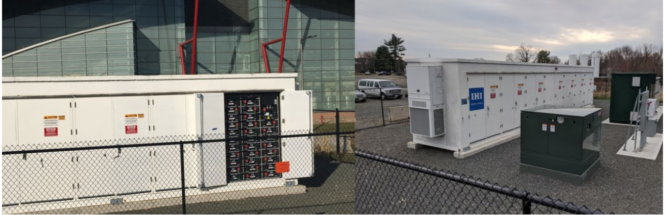
Figure 5. Battery Energy Storage System (BESS)
