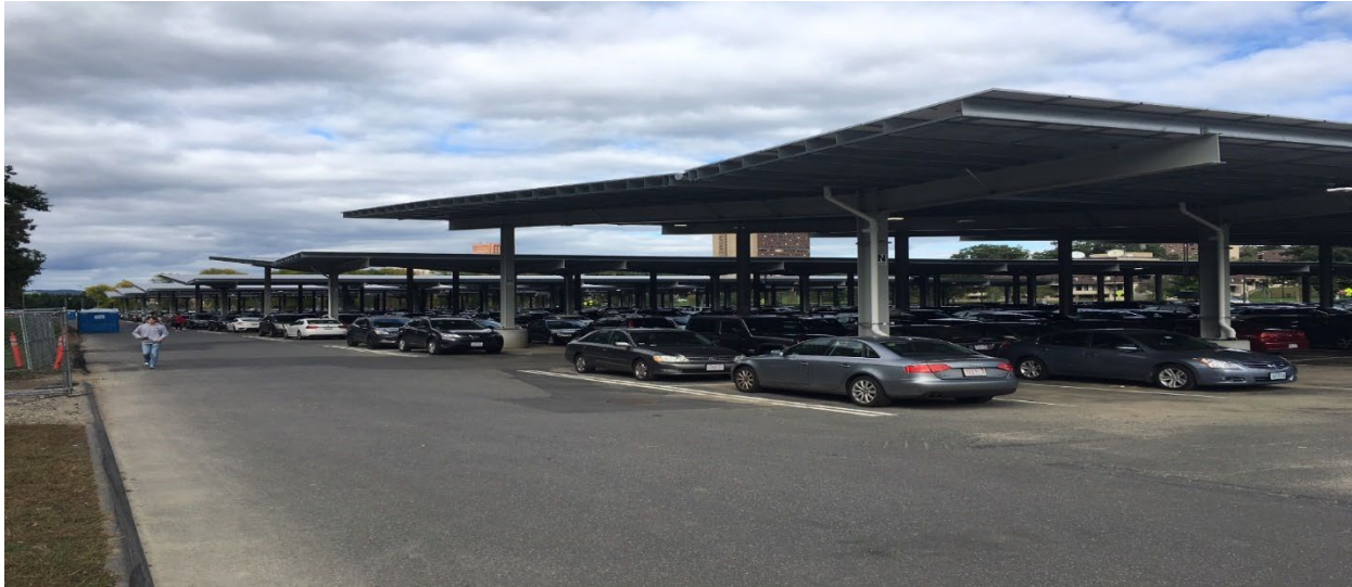
Figure 6. Lot 22 solar panels
