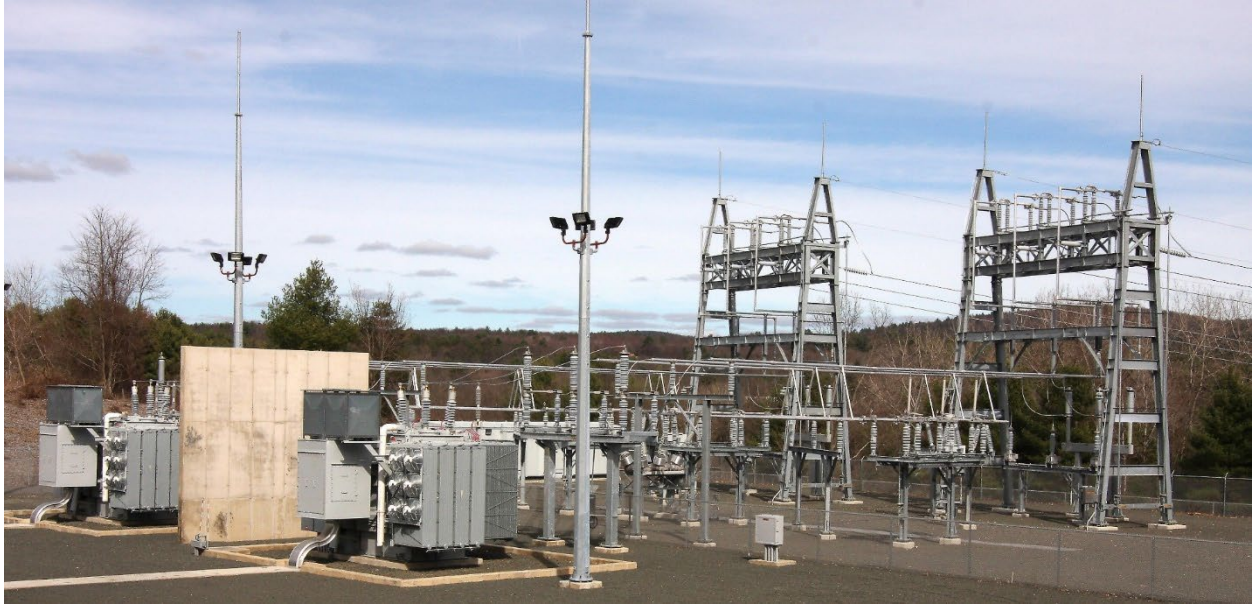
Figure 7. Tillson Substation (115 kV)
