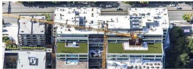
1101 Dexter installation with Firestone 30 year TPO and Firestone SkyScape Garden Roof. Contractor - Cobra BEC.
