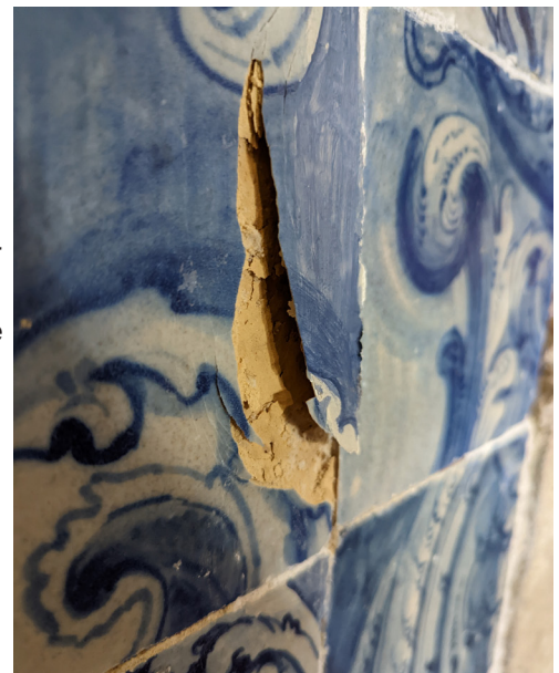
Ceramic tile flaking, likely due to the movement of water and soluble salts.
