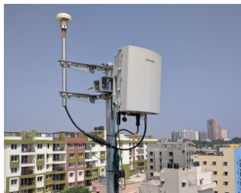
Figure 3. Small Cell situated in the terrace of a building in Bangalore, Karnataka
