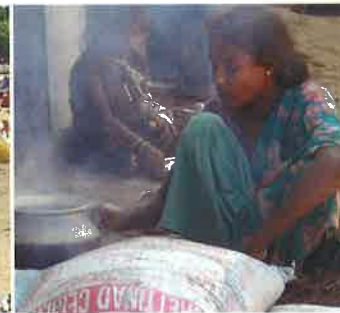
Life goes on around the installation of a Zenon Homespring unit in Nagapattinam, India. Photo courtesy of Jonathan Lieberman of Zenon Environmental.
