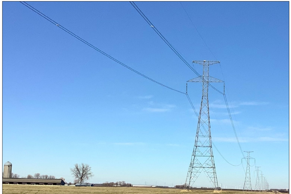
Photo of CU power line today, near Elrosa, MN [4] (taken by the author). HVDC lines have a characteristic two conductors at +/- 400 kV instead of the three for AC transmission. Each conductor here is actually two physical cables to carry more current.
