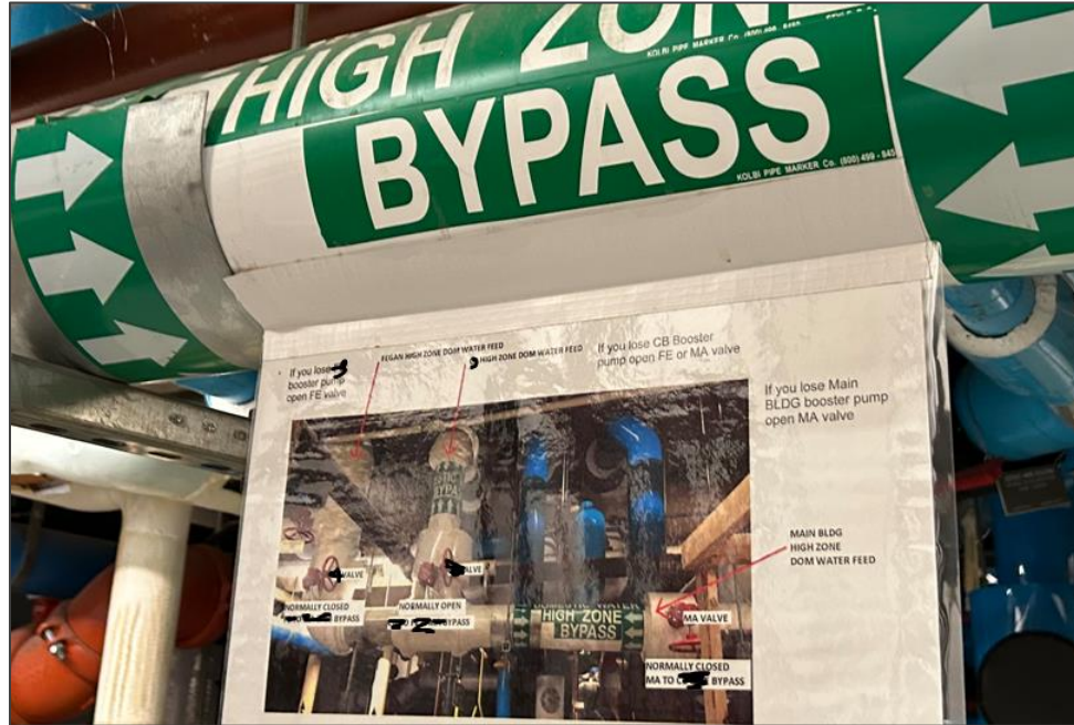
Properly maintained and labeled cross-connect (bypass)
