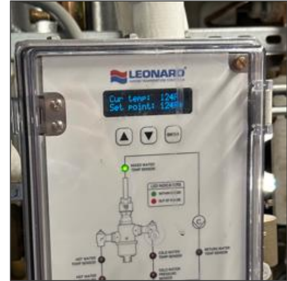
Proper water temperature on a mixing valve
