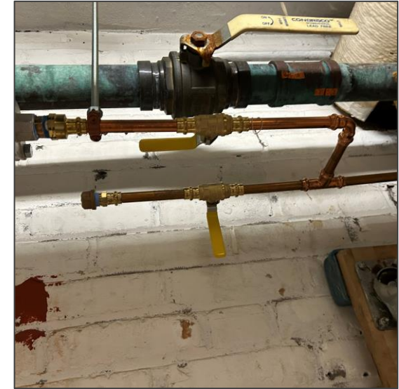
Dead leg piping
