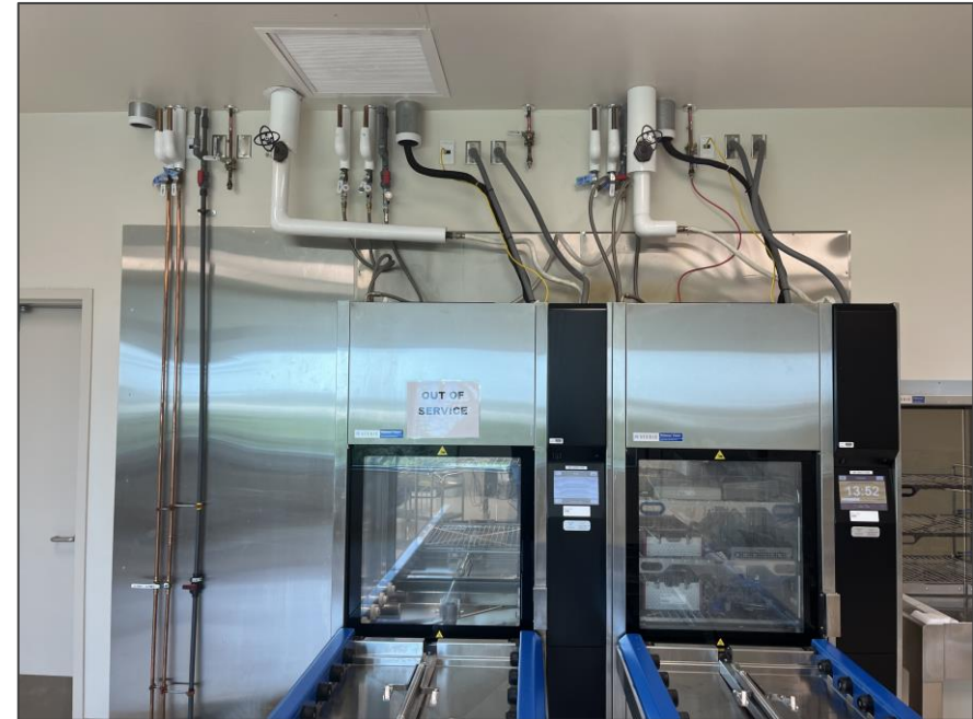
Dead legs for “future” washer/capacity (valve installed for flushing; piping later removed)
