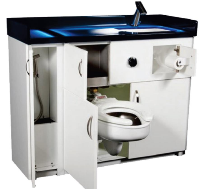
ICU Plumbing Fixture with dead legs
