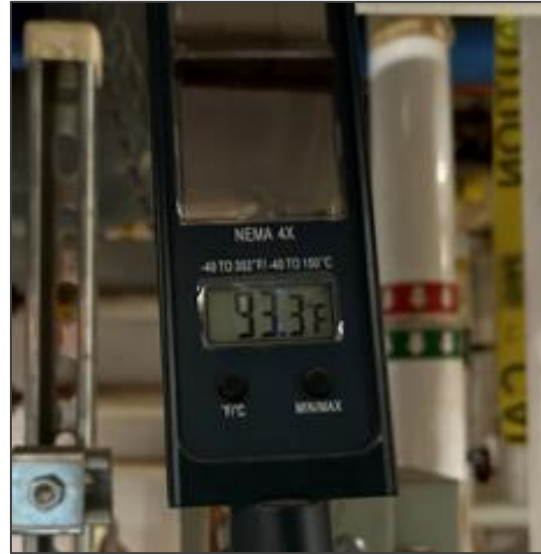
Mixed water heater <118 F (or malfunctioning)
