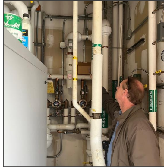
Dead leg piping
