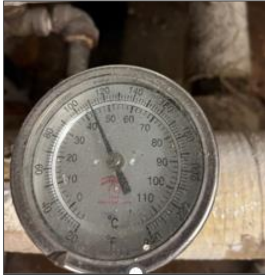
Hot water heater <140 F/Broken Gauge
