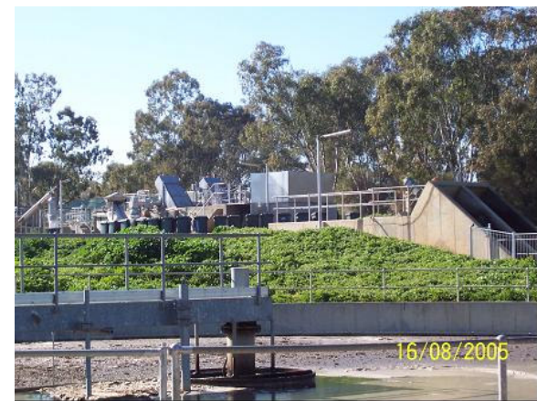
Photo courtesy Dubbo CC – Troy Junction STP
