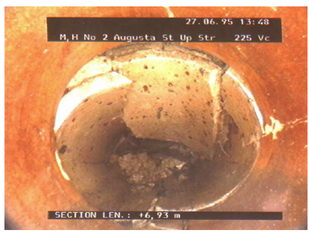
Source: WSAA Compendium sewer defects
