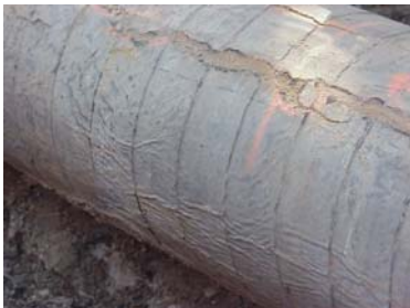
Defects in external coating
