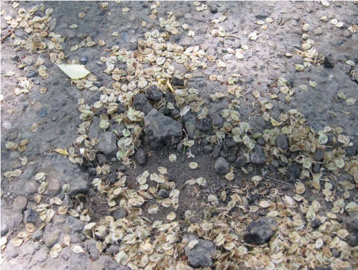
Photo 7: Example of Poor Pavement Condition
